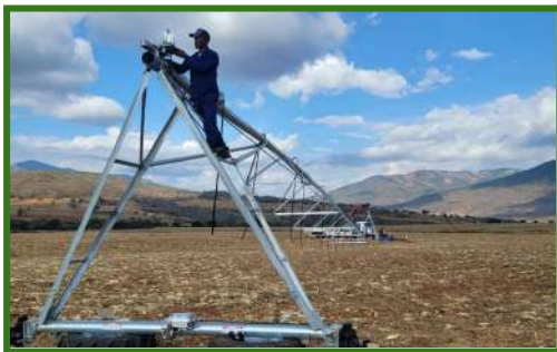
Pivot no 2 was installed at the farm.
